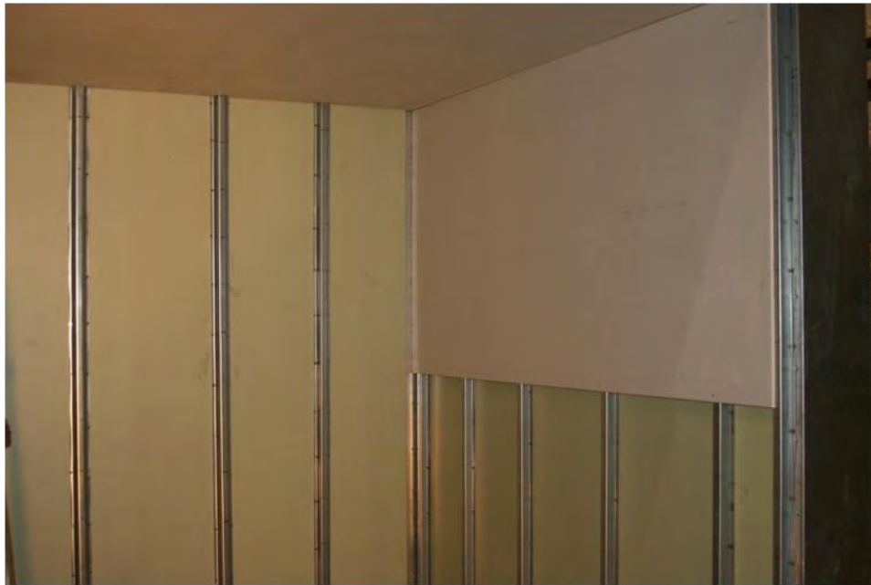
Figure 11. Walls with 1½-in. Furring Strips and Regular ½-in. Thick Gypsum Lining the Interior.
